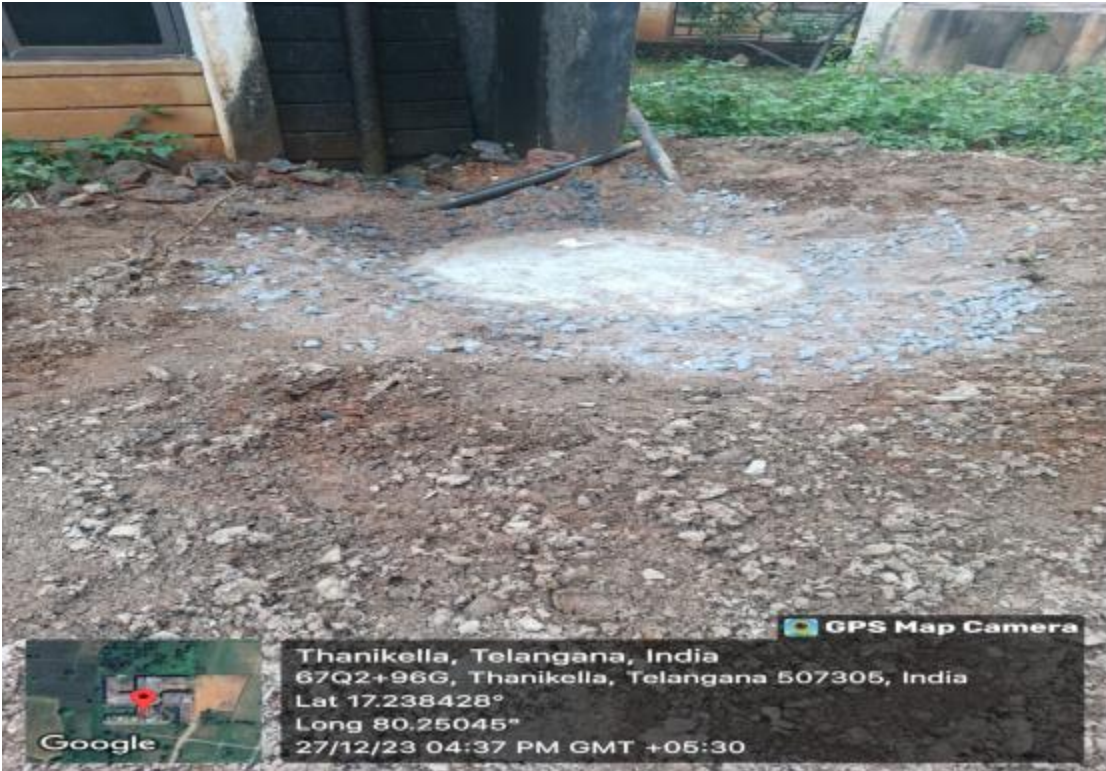
Rain water harvesting pit:
